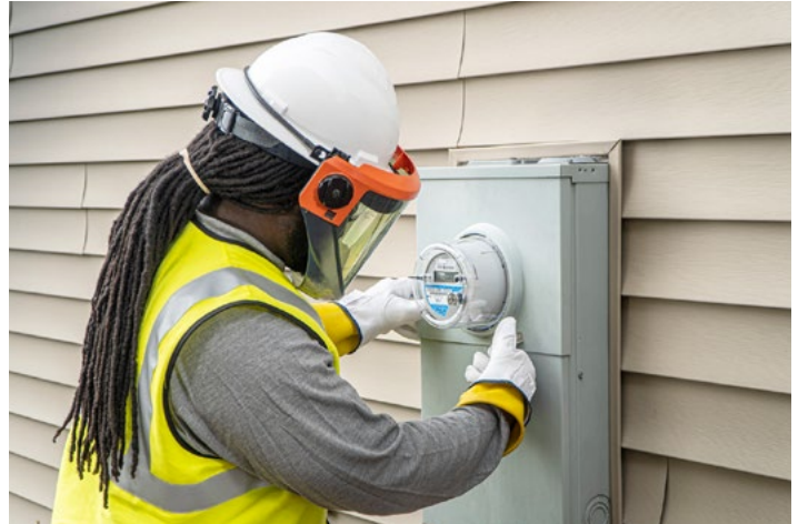
Smart meters like this one can be turned on and off remotely, permitting faster service and reducing service vehicle emissions.
