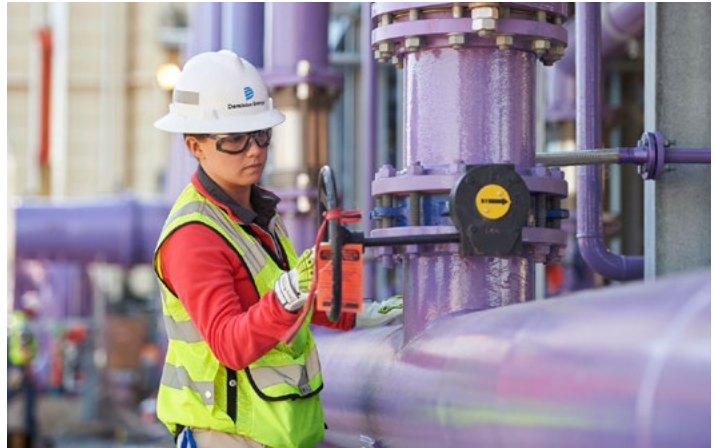
Workers at the Brunswick County Power Station produce electricity from clean natural gas, powering 340,000 homes and businesses.
