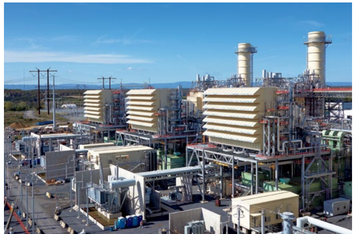
Warren County Power Station.
