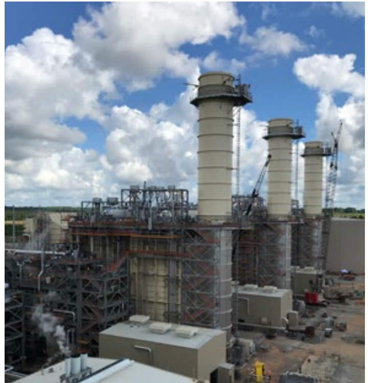
Greensville Power Station.
